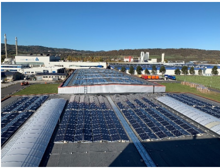
Some 1,725 MWh of solar power a year are going to be produced on 16,000 m 2 in future. (Source: Gebrüder Weiss)
