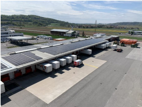
On the grid after a construction period of two and a half months: 5,922 panels were installed in total. (Source: Gebrüder Weiss)
