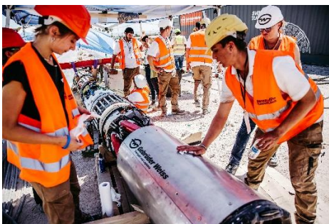
Caption: Groundhog Alpha, the Innovation Award-winning tunnel boring machine from Swissloop Tunneling (Source: Gebrüder Weiss)
